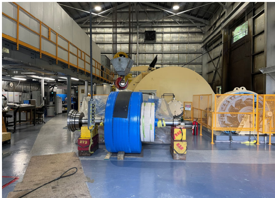
Phase 1 – Upgraded 2,250 hp motor
